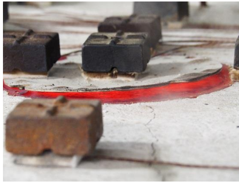
Figure 9. A photo showing the lift-up of the cap of the non-insulated opening and the glowing surface below it.
